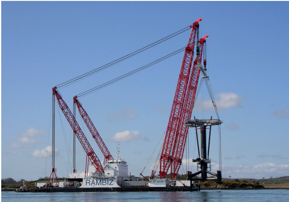
■ Photo 3 : Rambiz crane-barge installing the Seagen stream turbine on the Strangford Narrows site, Northern Ireland (© Marine Current Turbines, UK).
